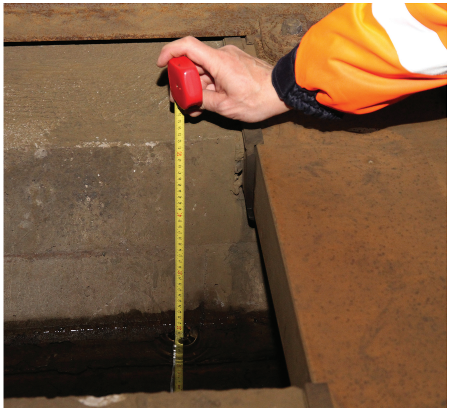
Standing water in the longitudinal groove of the mass-spring system (MSS) section, water level approximately 20cm
